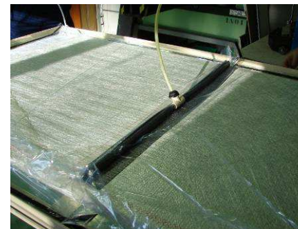
Spiral tubing put above a panel junction
